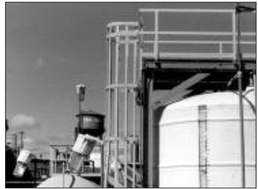
Fiberglass ladder cage assembly provides worker safe access to an outdoor platform.
