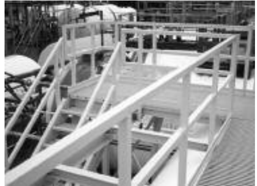
Handrail is used on walkways and platforms for safe maintenance free worker access.
